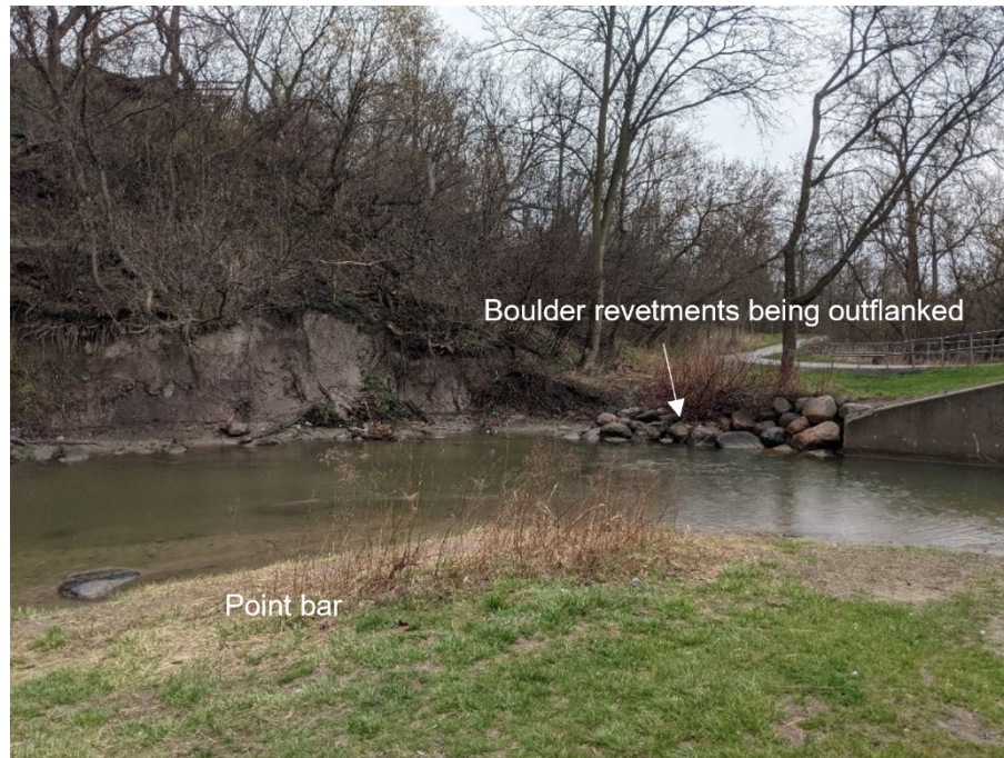
Photo 7. Bank revetment upstream of pedestrian bridge being outflanked at the downstream limit of an erosive scarp, along the Site 3 valley wall contact. Downstream view.
