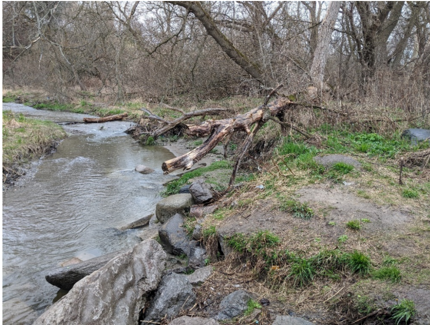
Photo 10. Riprap bank revetment at Site 8 that protects the Bike Path and left abutment of the Thomas Street bridge. Upstream view.
