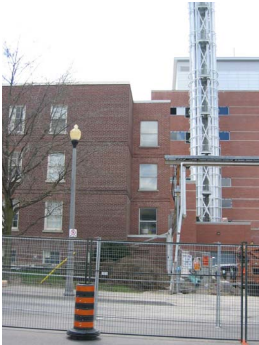
6. McLaughlin Hall, South West façade (showing addition that links McLaughlin Hall with Lakeridge Health Oshawa. April 2006
