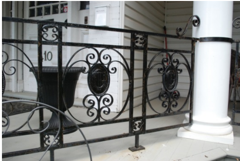
Black Metal Railing featuring the GT symbol in the centre.
