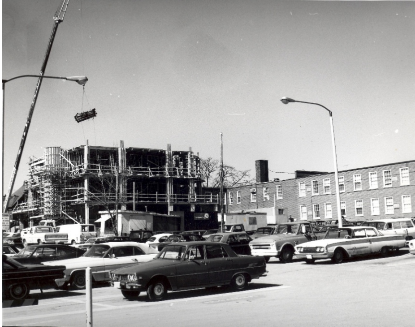
Figure 10- Looking roughly North-West at the Oshawa Clinic tower addition from the clinic parking lot off the West side of Charles St. Image: Thomas Bouckley Collection, RMG. 1970
