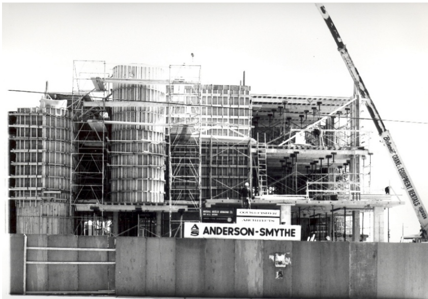
Figure 9 - Looking South at the front of the Oshawa Clinic tower addition on King St E. There are signs saying that Ogus & Fisher are the architects and Anderson-Smythe are the contractors, and a crane on the right side of the photograph. Image: Thomas Bouckley Collection, RMG. 1970.
