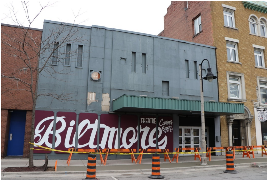
Figure 12 - 39 King Street East, Test Spot on Stucco by owner. April 2021, Photo Courtesy Robert T. Bell
