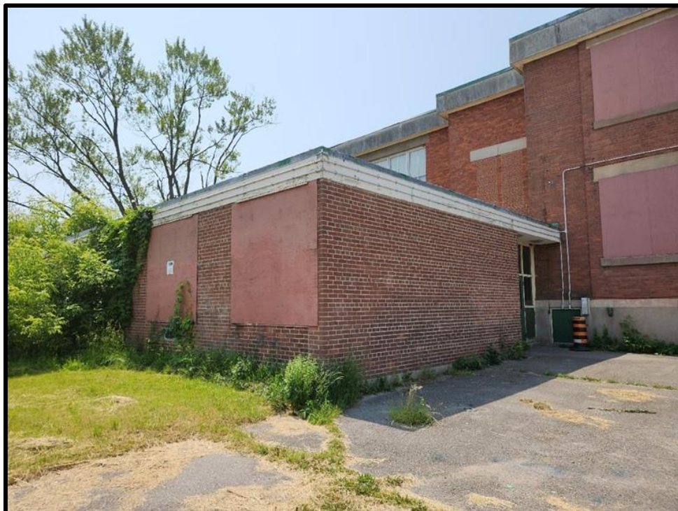
Image 6: Northeast Corner of Rear Addition at 827 Gordon Street (Photo taken June 19, 2023; Facing Southeast)
