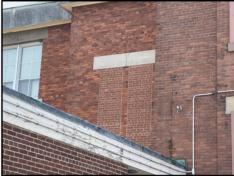
Image 17: Detail View of Altered Openings on Rear Elevation of 827 Gordon Street (Photo taken on June 19, 2023; Facing East)
