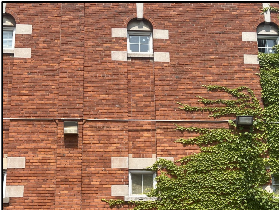
Image 14: Detail View of Arched Window Openings at 827 Gordon Street (Photo taken on June 19, 2023; Facing North)
