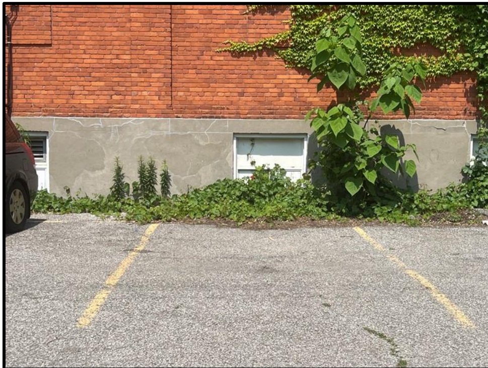
Image 16: Detail View of Foundation at 827 Gordon Street (Photo taken on June 19, 2023; Facing Southeast)
