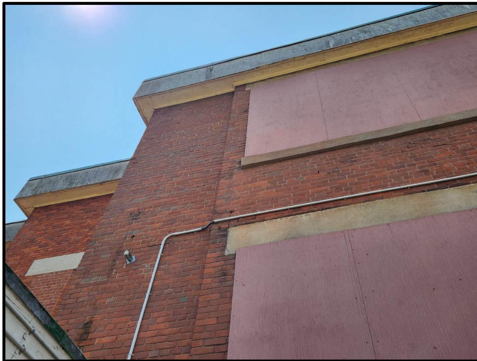
Image 18: Detail View of Altered Parapet on Rear Elevation of 827 Gordon Street (Photo taken on June 19, 2023; Facing East)
