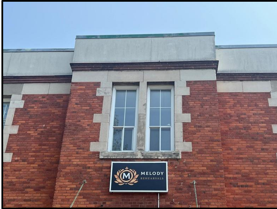
Image 11: Detail View of Parapet and Window Surround at 827 Gordon Street (Photo taken on June 19, 2023; Facing Northeast)
