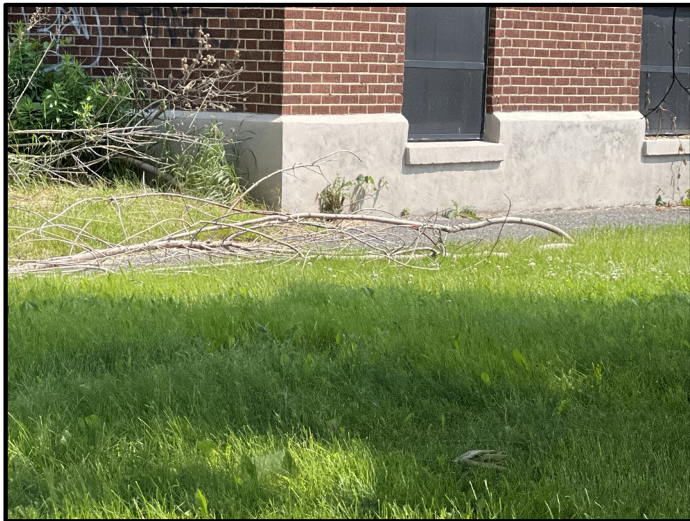
Image 8 Detail of Foundation at 149 Harmony Road South (Photo taken June 19, 2023; Facing Northwest)
