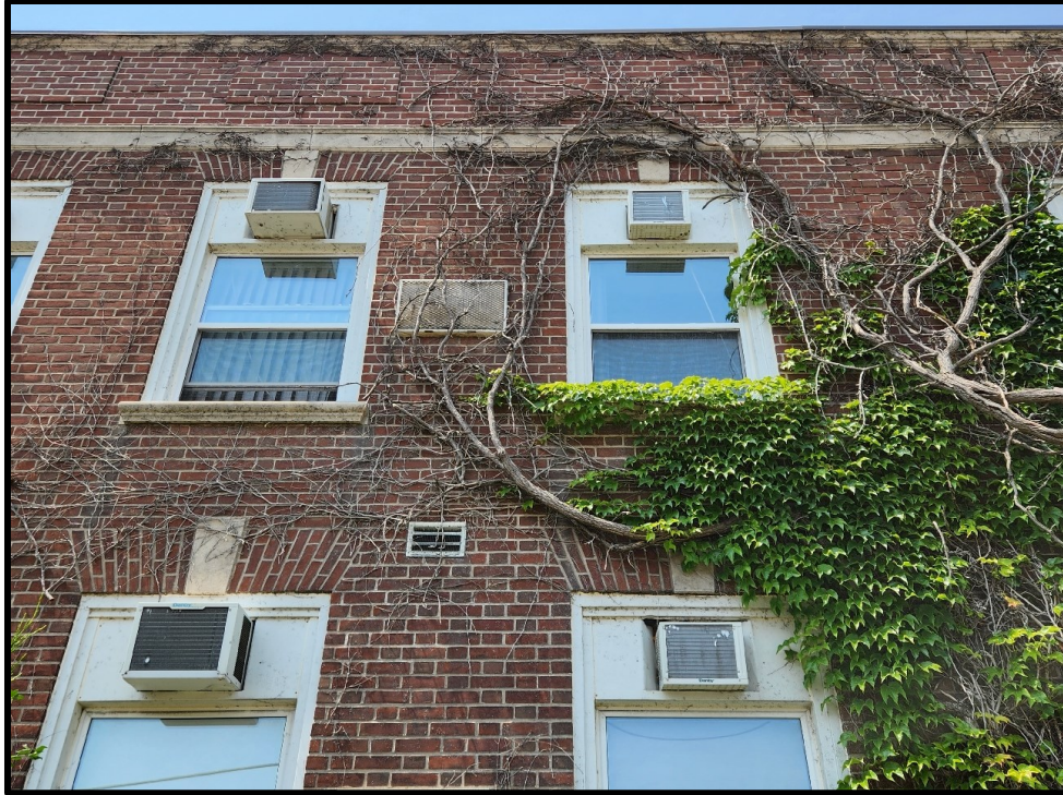
Image 7: Detail View of Window Openings with Keystone Flat Arch and Cavetto Mould of 1948 East Wing (Photo taken on June 19, 2023; Facing West)
