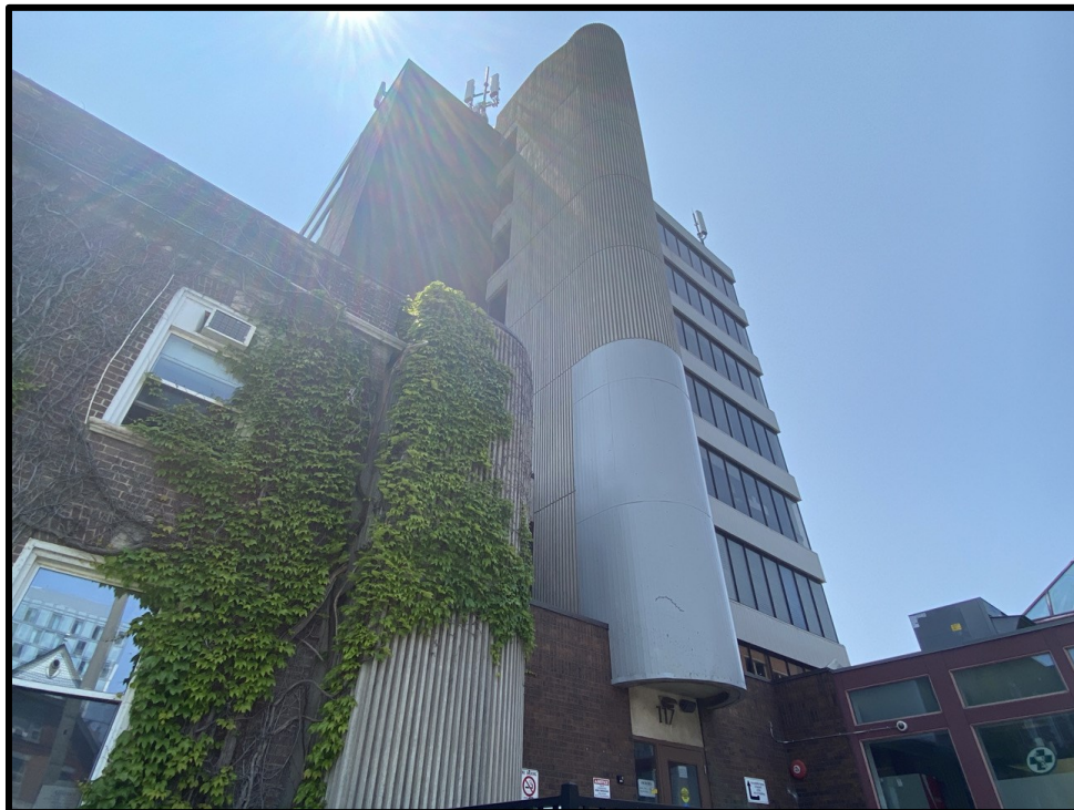
Image 10: Detail of Rendered Concrete Extension on North Elevation of 117 King Street East (Photo taken on June 19, 2023; Facing South)
