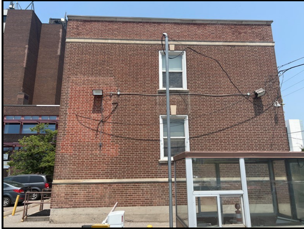
Image 5: South Elevation of 1948 East Wing of 117 King Street East (Photo taken June 19, 2023, Facing North)
