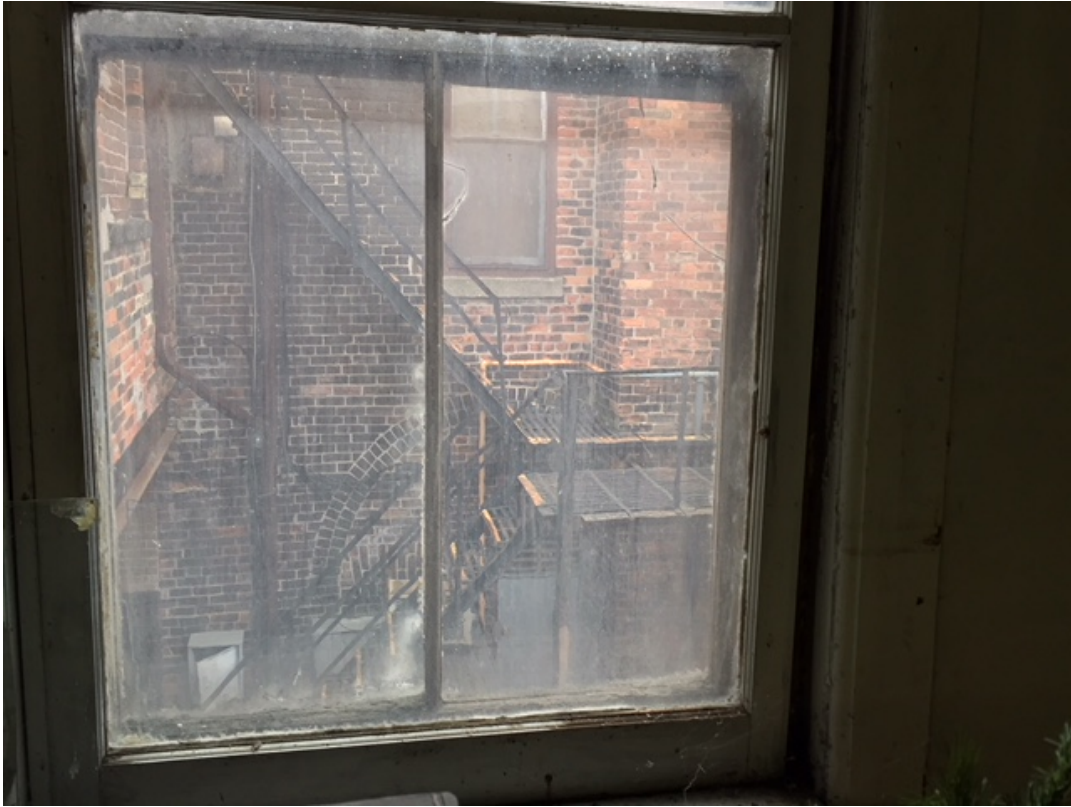
3. View out the south east window, note the brick archway on the back of the Wilson/Lovell Building. This was a thruway at one time from King Street.
