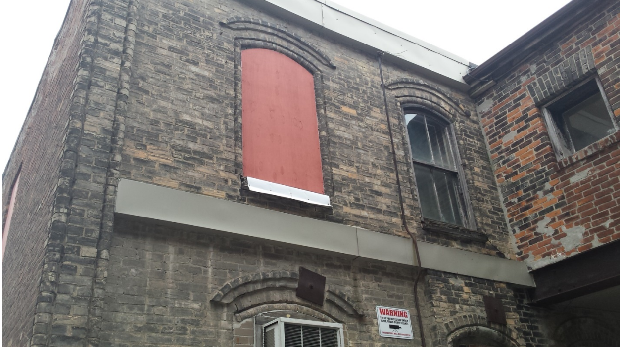
3. Carriage Shed, South Façade, close-up of window details and moulded brick on south east corner, 16 King Street East
