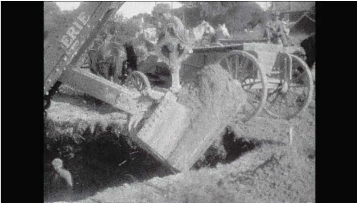
Figure 7: Foundation being dug by the Erie Steam Shovel Company. Source: Ted Rundle
