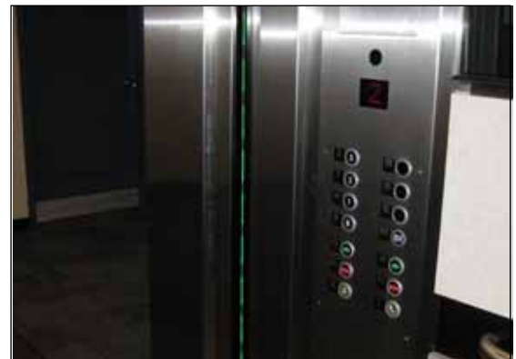
Elevator sensor door and floor registration buttons.
