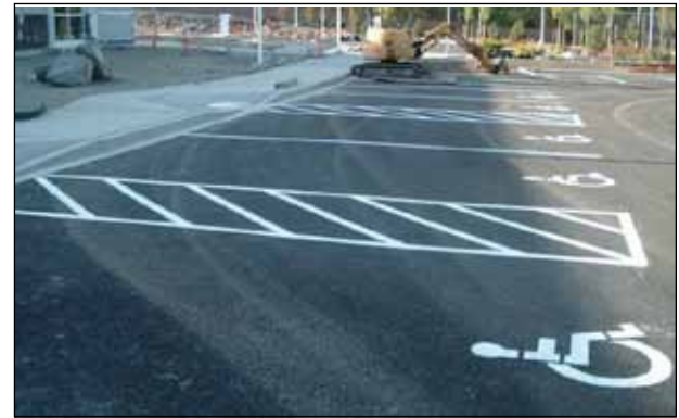
Accessible parking spaces with access aisle and curb ramp. Source: Taken from "Illustrated Technical Guide to the Accessibility Standard for the Design of Public Spaces" by GAATES, 2014, p. 115.
