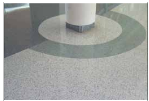
Where a structural column / support may be within an accessible route, a colour contrasted floor surface at base helps identify its location to prevent a potential bumping hazard.
