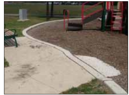
Curb ramp into play space where there is a level change between accessible route and play space.
