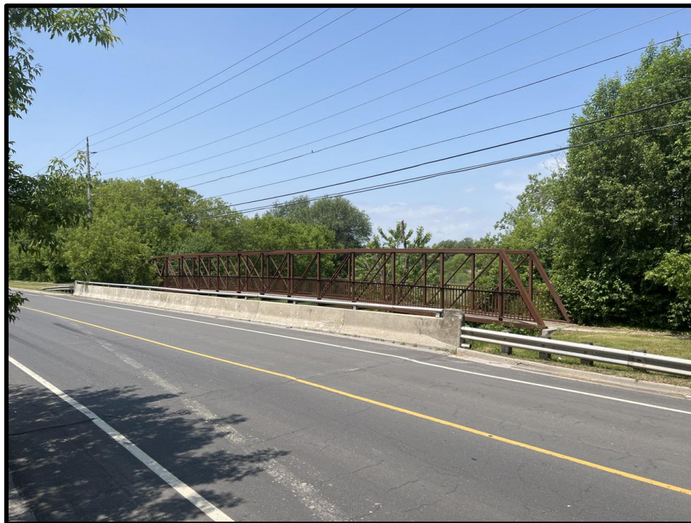
Image 6: Pedestrian Bridge Over From South Side of Col. Sam Drive (Photo taken June 13, 2023; Facing Northwest)
