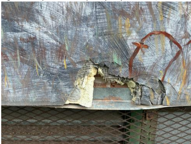
Figure Thirty-two: "Camp X" (Tony Johnson, 100 Simcoe St. South) – South impact damage
