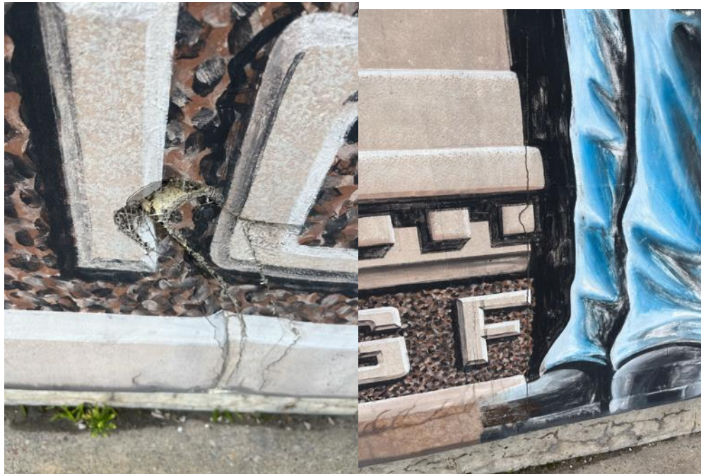
Figure Sixteen: "Oshawa's Development (Historical Industry and Development)" (Robin Burgesse, Go Bus Station, 47 Bond St.) – Impact Damage and cracks
